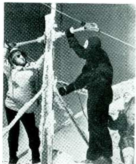
Messrs. Cody, Wiggin, and Corwin erect the television antenna in a 77-mile wind atop the weather observation station
