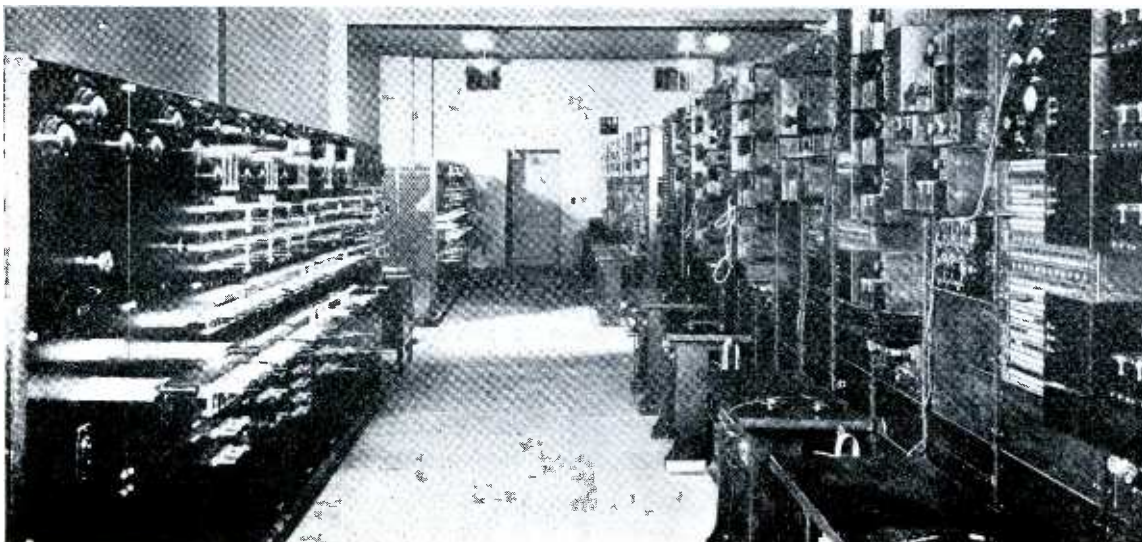
Amplifier room of a modern sound studio. Amplifier equipment for eight recording channels is shown at right with power control panels at left. Estimated cost of the total electrical equipment involved, $1,000,000.
