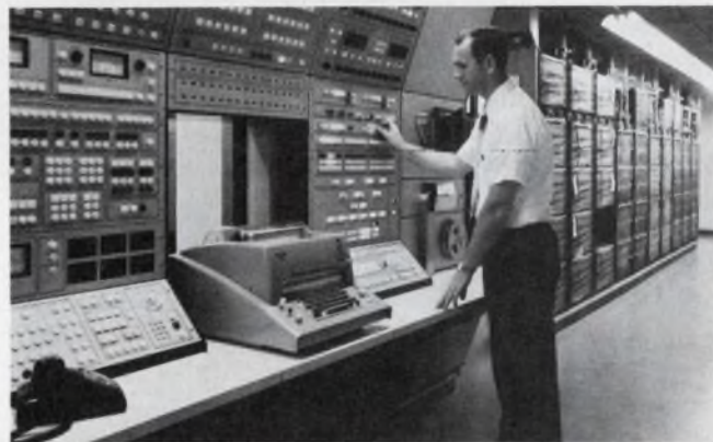
Stored program computer control makes customer service changes a matter of issuing instructions to a computer. The computer performs extensive monitoring in GTE Automatic Electric's Electronic Automatic Exchange. Sealed reed switches complete the circuit paths; dual processors ensure reliability.
