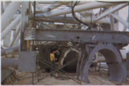
Welding habitats , such as Taylor's, are lowered to the ocean floor, where divers, monitored by transducers and TV, descend in bells to weld pipes.
