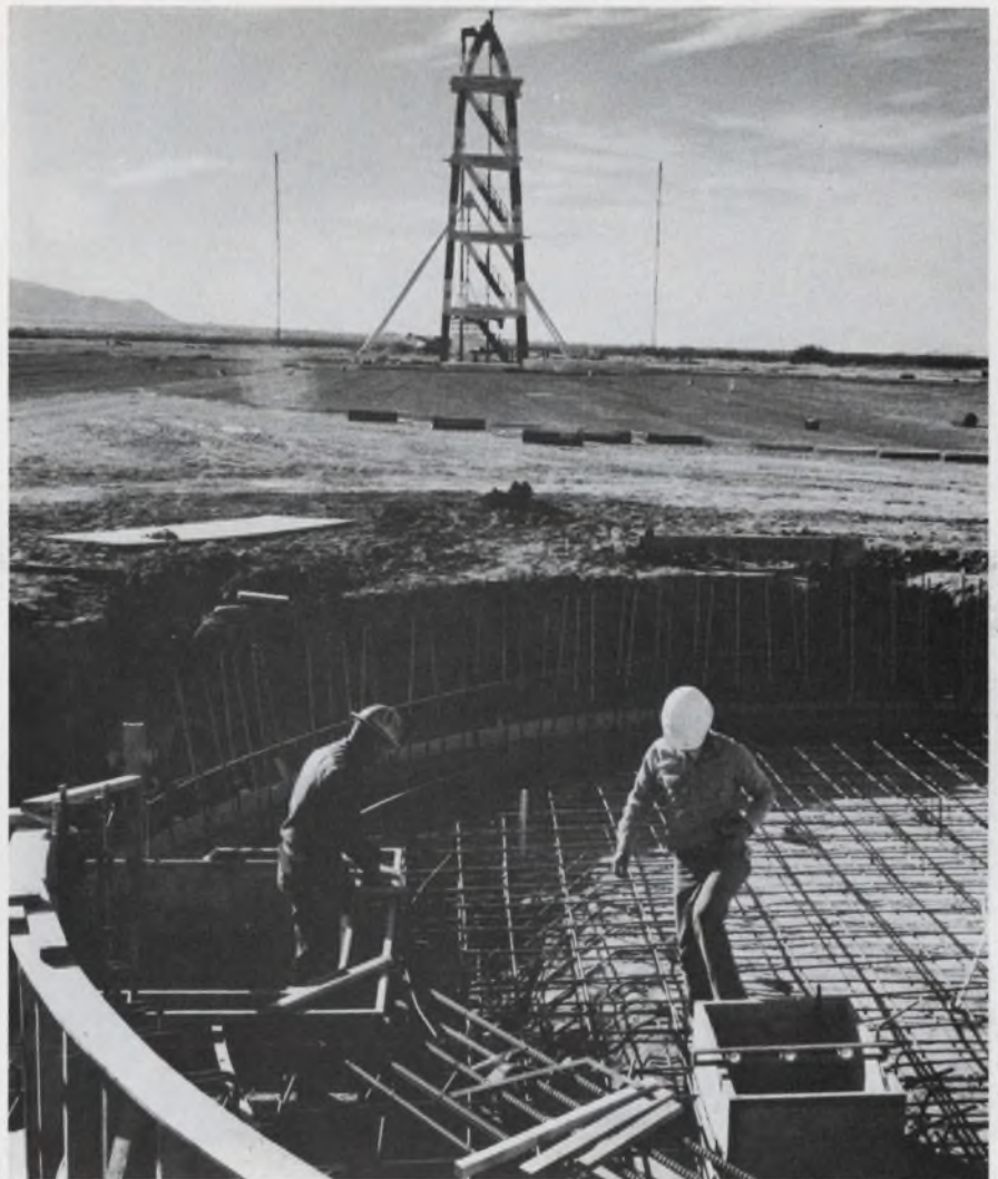
When this turntable is completed, vehicular radio antennas will transmit to five receivers in the 100-foot tower 500 feet away. Buried steel-wire mesh will provide a swamplike or saltwater environment to the transmission.
