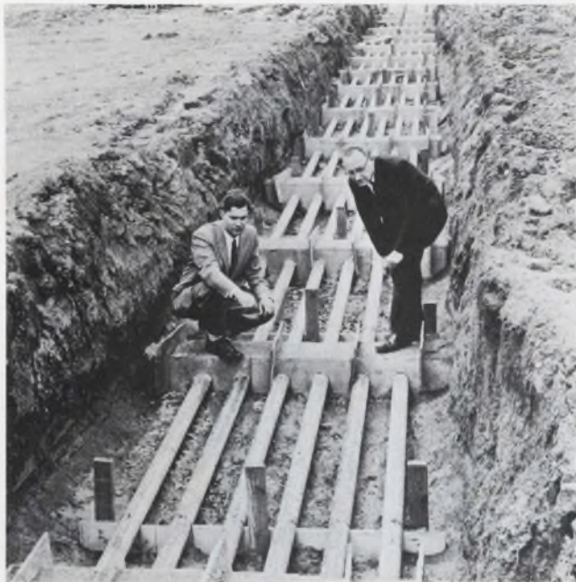
Millimeter waveguide is coming. Circular guide will be used for its low loss characteristics. This experimental installation is at Bell Labs, Holmdel, N. J.
