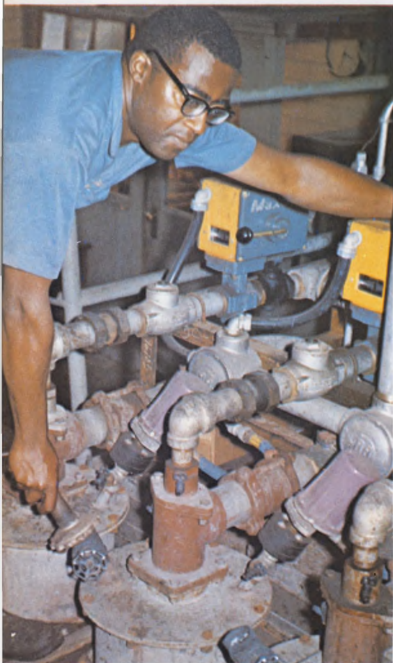
This man is lighting a methane burner with a high-voltage wand at Philadelphia's old N.E. Sewage Treatment Plant. A thermocouple used to be used to ensure ignition of the flame, but heat damaged the sensitive junction. Nine years ago the plant replaced the thermocouples with ultraviolet sensors housed in the purple cylinders (lower right corner of photograph). Should the gas fail to ignite, the sensor triggers a valve, which prevents the flow of raw methane.
