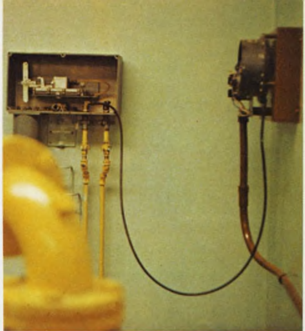
This differential-pressure sensor blew its diaphragm. A Honeywell representative was said to have ordered three replacements but when they arrived with a bill for $375, he returned them to their manufacturer.
