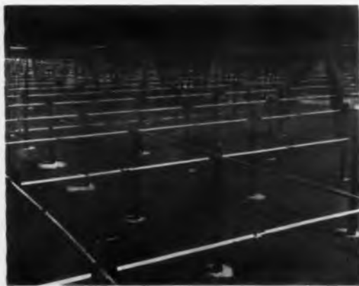
Acres of antenna being constructed by NBS and the Instituto Geofísico de Huancayo, Peru, will be used in conjunction with a 6-mw transmitter for ground-based exploration of space. A total of 9,216 crossed dipoles covers 22 acres.
