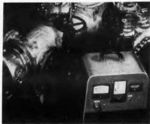
Portable ultrasonic flowmeter uses transducers mounted on opposite sides of pipe insert to measure quantity and rate of flow. The unit above, a meter readout and direct writing recorder, checks a water meter
