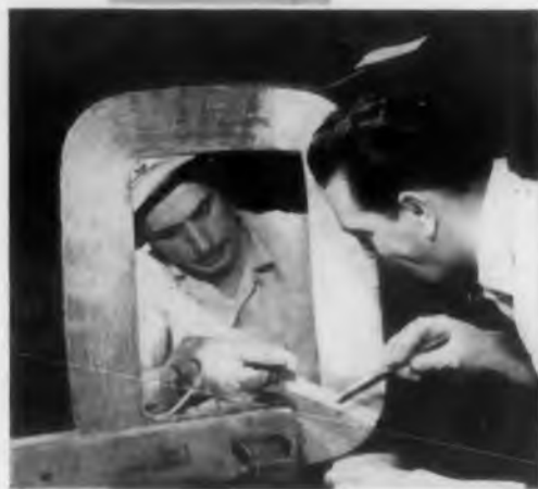
Applying Epon resin sealing compound, formulated by EpoxyLite Corporation, El Monte, California, to a 400-kva transformer winding at Larsen-Hogus Electric Co., Los Angeles, Calif.
