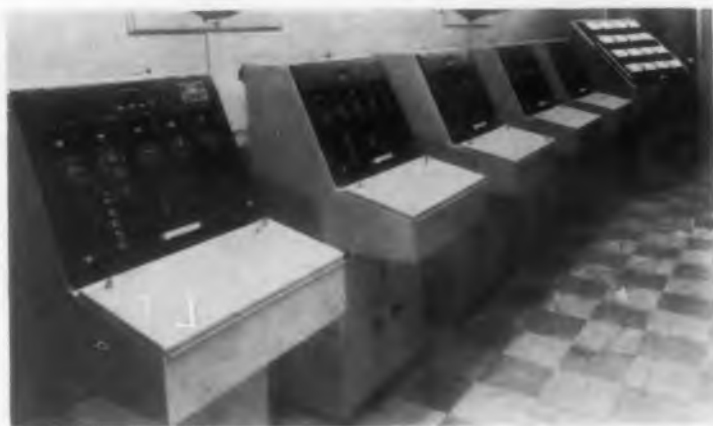
Monitor consoles for TACAN Data Link. System can be answer to air traffic control problems.
