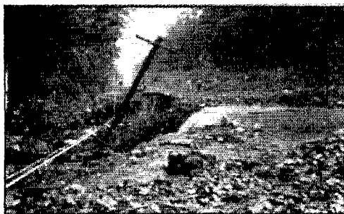
This is the type of flood washout that took communications with it at Ithaca, N. Y., in 1935.
