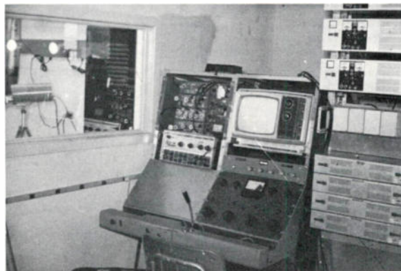
Control console for Globe-Miami, Arizona system built by Clyde Fette built out of materials at hand.
