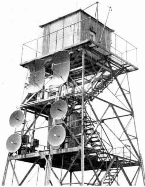
Figure 13. Top of Neshanic, N. J. tower, showing tower house, television and diversity antennas, and wave guide antennas installed for 6000-mc experiments
