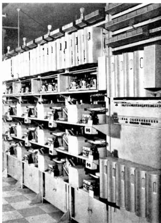
Figure 4. Varioplex Central Office equipment with control rack in foreground.
