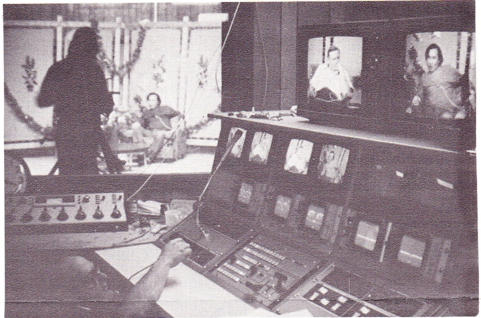
KYUK-TV, BETHEL, ALASKA . . . above is shown a partial view of the Sparta A-20B audio console flanked by TV Control. Engineer Bob Tinkle is nearly under the table (lower left) making some equipment adjustments. —Bennett Engineering Associates Photo
