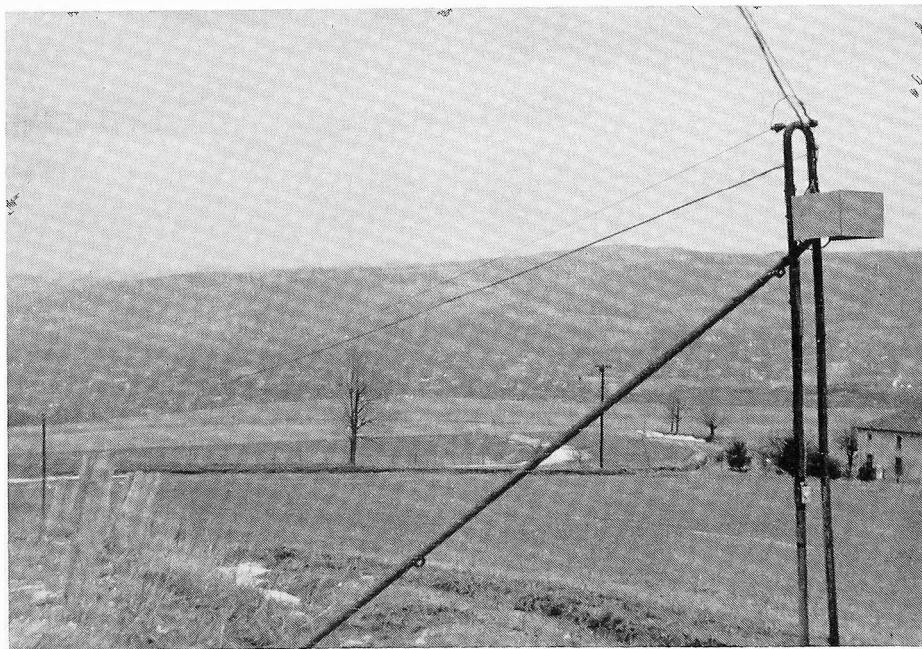
Fig. 5. Distribution Amplifier Mounted on Utility Pole. (Photograph by courtesy of Taco Antenna Co.)
