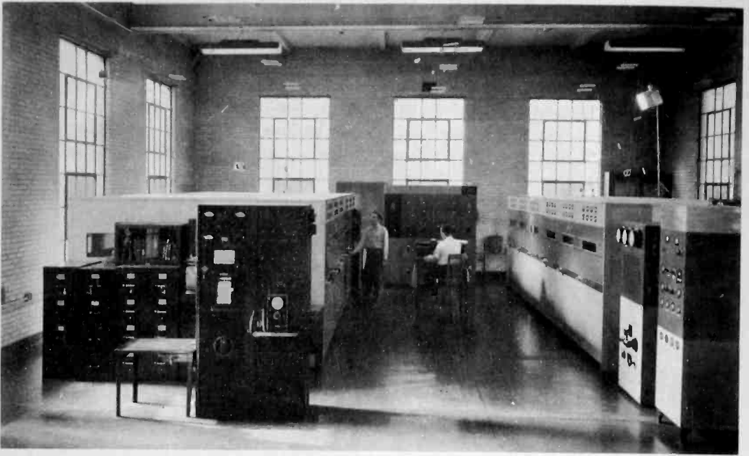
Figure 16. Interior of NBS Radio Broadcasting Station WWV. The banks of six transmitters are carefully monitored and precisely controlled to generate signals with an accuracy of two parts in 100 million.
