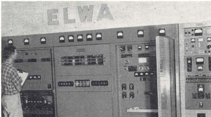
Gates HF-10B 10 KW transmitter with associated equipment.
