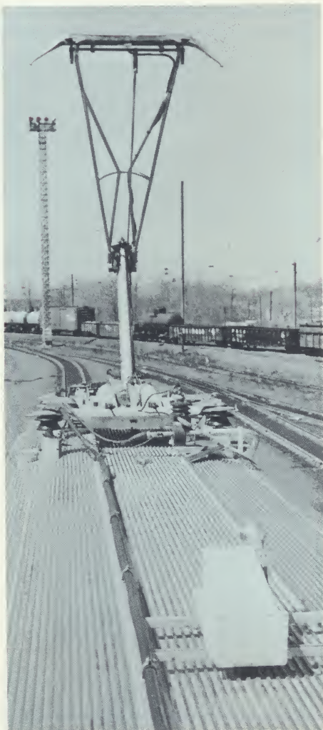
Enclosed in a weatherproof housing (foreground) an Ampex closed circuit television camera is used to monitor the pantograph at the center of the picture. Pantograph's motion is recorded on one of two on-board Ampex VR-7000 portable videotape recorders.
