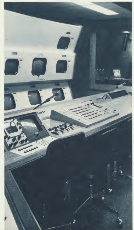
Control room for studio 1 (40 by 60 feet) where Scarborough College produces its extensive lecture series. It is easily the match of many commercial facilities. Audio control room at right includes an Ampex AG-440 recorder and Ampex 620 speaker amplifier.
