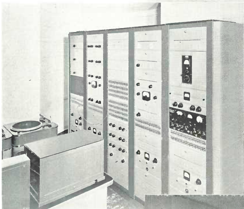
A partial view of the master control installation at WCAO, Baltimore, Md., showing the rack-mounted audio equipment. This is companion equipment to that shown on the opposite page top view.
