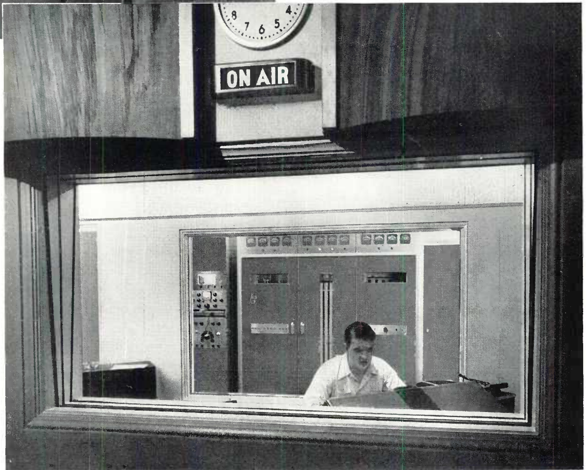
Three kilowatt FM transmitter, Type BTF-3B, as viewed from studio B, at WATG-FM, Ashland, Ohio.
