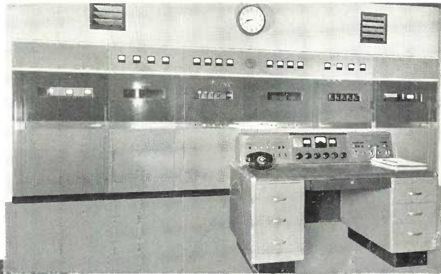
Installation of five kilowatt transmitter, Type BTA-5F, at KGKL, San Angelo, Texas. View shows left and right wing extension cabinets which contain broadcast audio and antenna phasing equipment.
