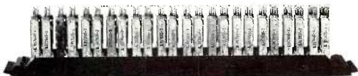
A Rear View of the 33-A Jack Panel
