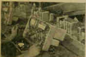
Interwiring of component parts inspected.
