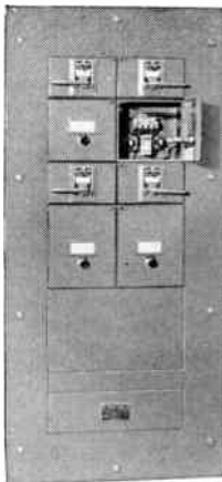
QMB Motor Starter Switchboard
