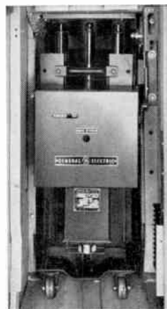
Breaker lowered, ready to be rolled out
