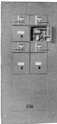
QMB Motor Starter Switchboard
