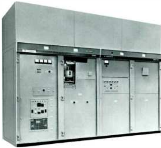
SW-50 with heat exchanger [front doors removed]
