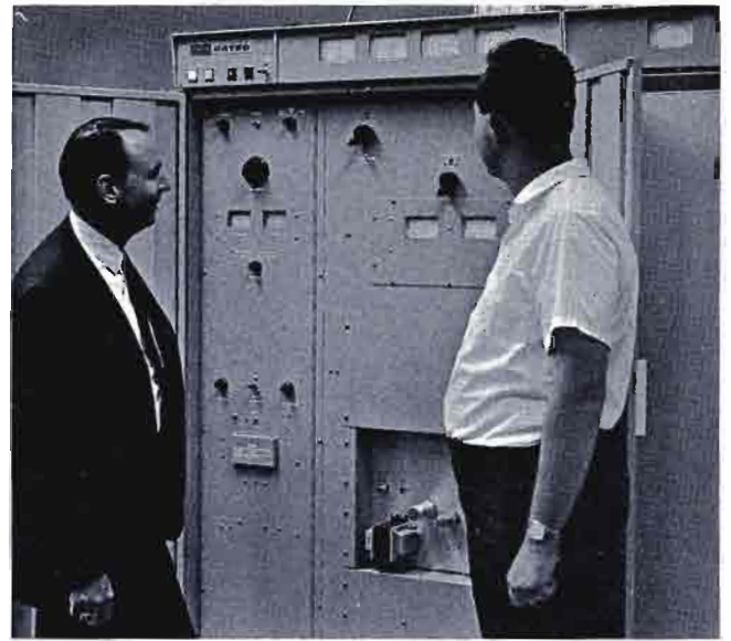
WGAN-FM, PORTLAND, MAINE —Utilizes a Gates 40 kW FM transmitter (two 20 kW transmitters with combiner and common exciter).
