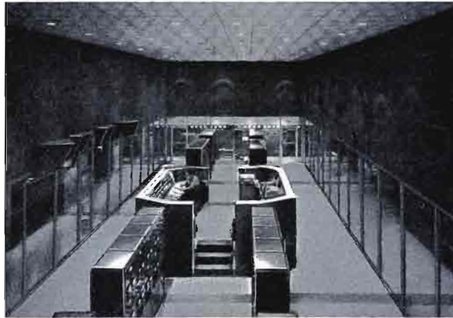
VOICE OF AMERICA —Six Gates 50,000 watt Model HF-50C transmitters in use at the Greenville, N. C. transmitting station.
