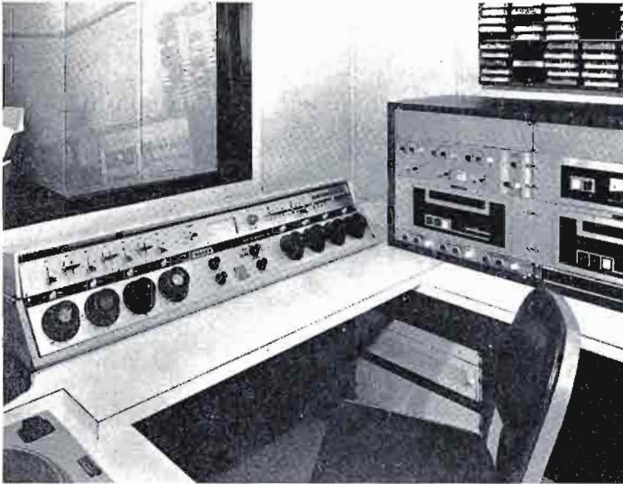
GATESWAY II CONSOLE AND CARTRIDGE TAPE EQUIPMENT WEEL, BOSTON
