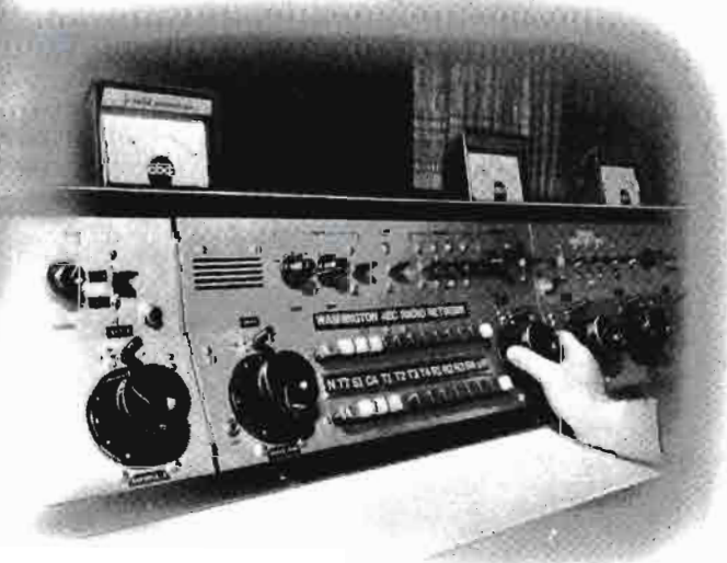
"CONTROL CENTER" WASHINGTON, D.C.
