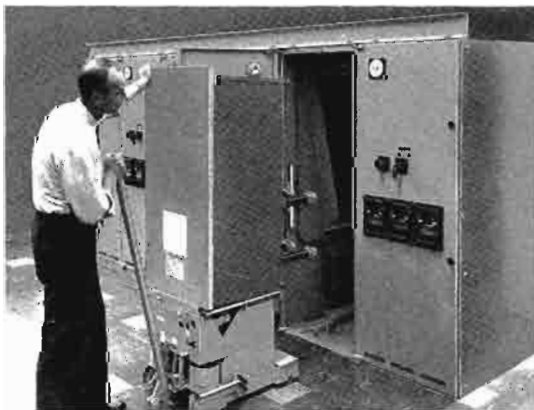
One of several 4160 volt primary power breakers with 150 megavolt ampere rating.
