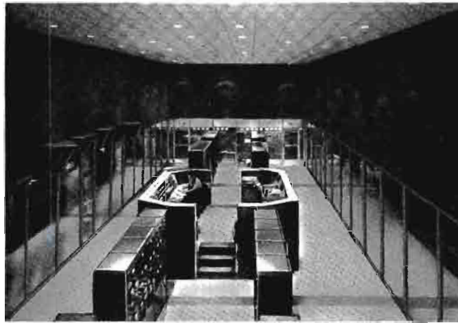
VOICE OF AMERICA—Six Gates 50,000 watt Model HF-50C transmitters are in use at the Greenville, N.C. transmitting station.
