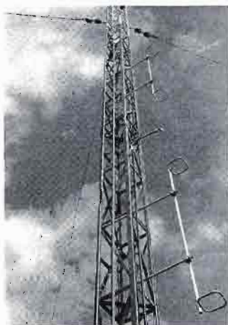
RA-4 Base Station Antenna.
