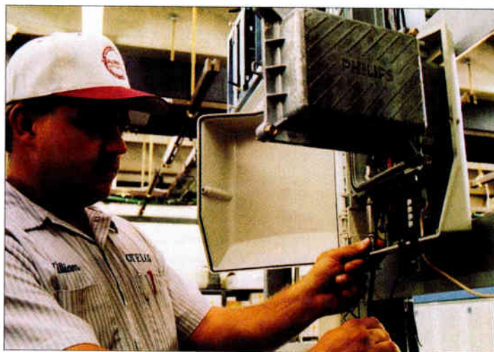
Otelco service technician William Blythe examines an HFC telephony subscriber interface unit (SIU) in the central office. This SIU is connected to the HFC network, enabling Otelco to use the in-house unit to test the telephony system's performance.
