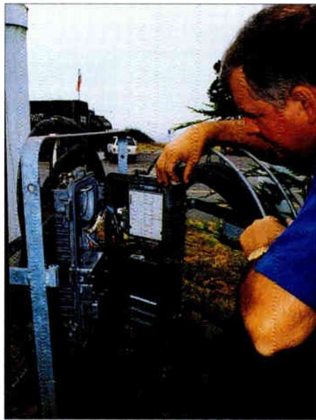
Mike Cline, general manager of Century Communications' Mendocino County, Calif. system, inspects a Philips node in preparation for the installation of a fiber optic backbone to support "Distance Learning Television."
