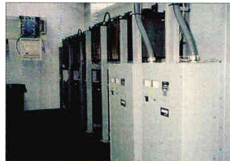
Figure 4. Battery powering for grooming facility
