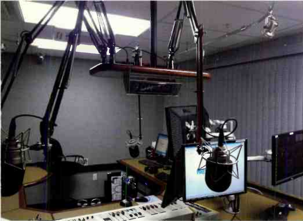
Detail of the suspended mic boom mounting platform
