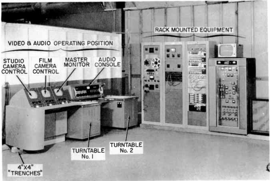
Fig. 8-3. Temporary "In-Plant" Training Setup of Doge TV.
