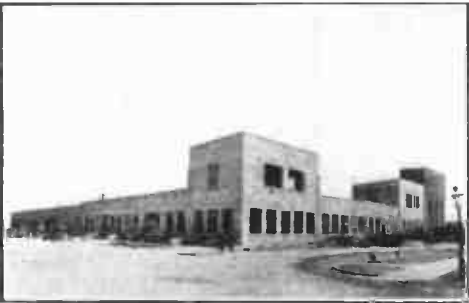
Plant No. 7, nearing completion, adds 50,000 square feet of space and will employ 1000 more men and women.
