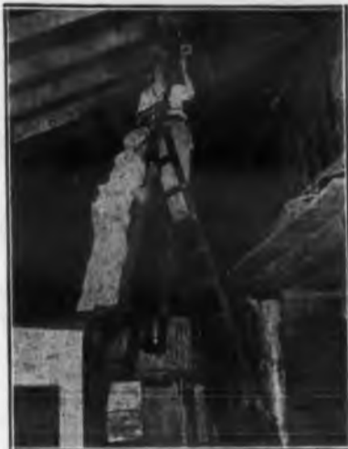
MEMBERS OF THE INTERNATIONAL BROTHERHOOD OF ELECTRICAL WORKERS spent many hours of freely given time installing the quaint and intricate system of lighting.
