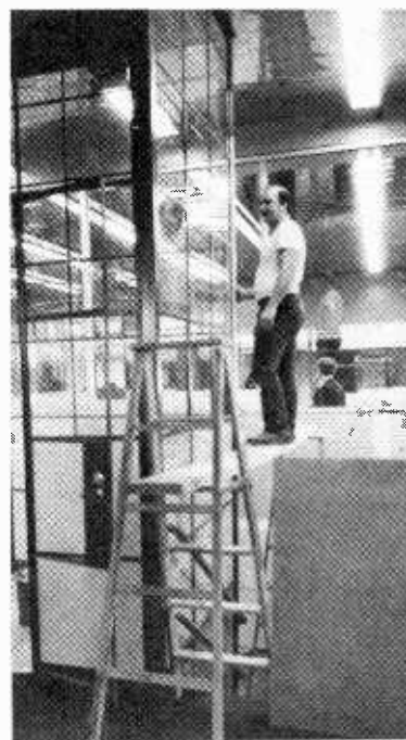
Best Of Booth Worlds. Construction worker, standing on a scaffold in the new New York Tower Records store's stairwell, puts finishing touches on one of the two DJ/VJ booths in the outlet. The other booth, for the classical and show sections, is located directly below the booth pictured. (Photo: Chuck Pulin)
