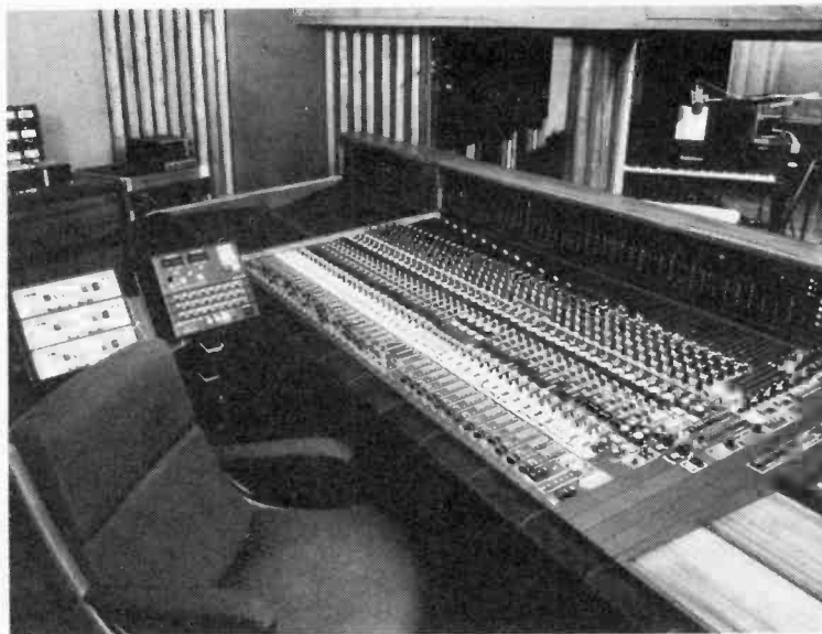
CONTROL BASE —The control room of the new CECCA Sound Studio in Dallas, showing the MCI console. The studio is owned by Charley Pride.
