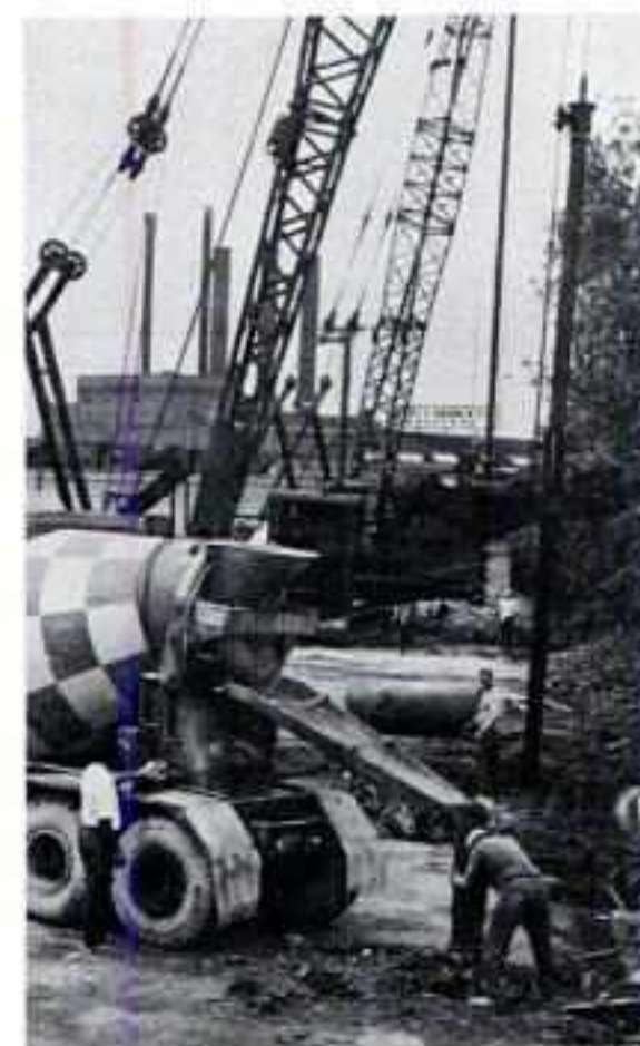
BALLY EXPANDS. This scene shows workmen commencing a 50,000-square-foot expansion of Bally Manufacturing Corp. building on Belmont Avenue in Chicago. This addition, according to Bally president, Bill O'Donnell, comes less than a year after the completion of another addition. Bally's complex will now extend back to the shoreline of the Chicago River. Bally's expansion reflects its international scope with shipments daily going to such countries as Japan, Australia, Europe, Israel, Lebanon, Kenya and Thailand and even to Iron Curtain nations. The new annex will be used primarily for basic fabricating, O'Donnell said, and assembly and inspection will be carried on in the present plant. O'Donnell said he is looking now for still more space in which to expand.
