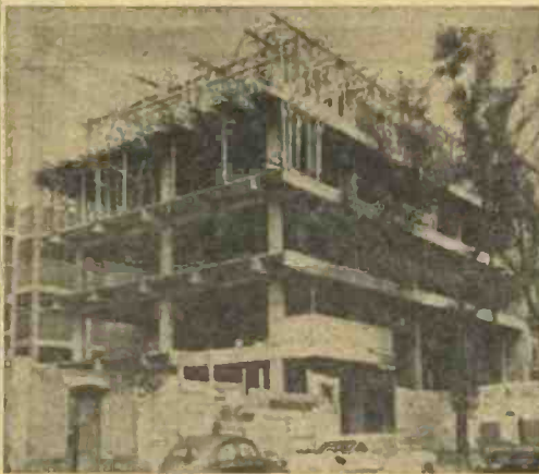
SCHEDULED TO BE COMPLETED by the end of September is Casa Riojas' $250,000 addition—a modern five-story, block-long building which will house offices, showrooms and warehouse. Production will continue in the old building.
