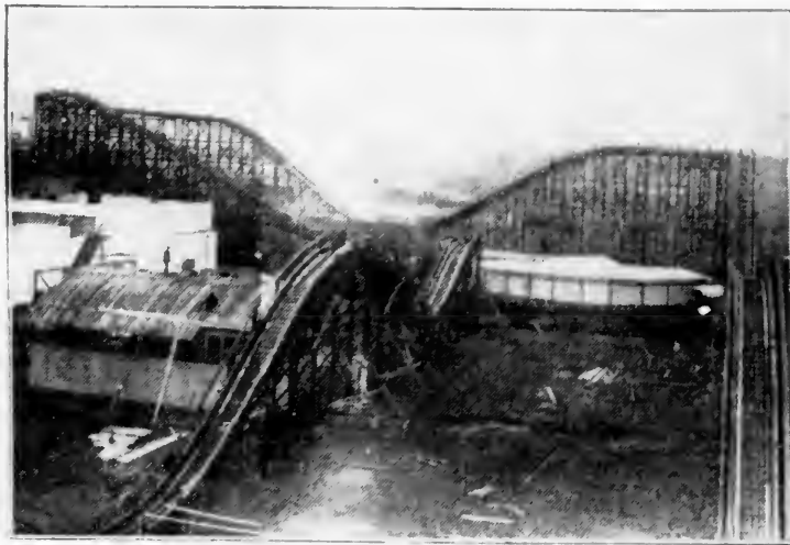
A view of the giant switchback in course of construction at the British Empire Exposition, Wembley Park, London, England.
