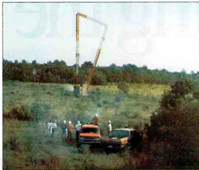
KLVI-AM/Beaumont, TX recently demolished and replaced three of its four broadcast towers as part of a $500,000 renovation of its transmitter facilities.
