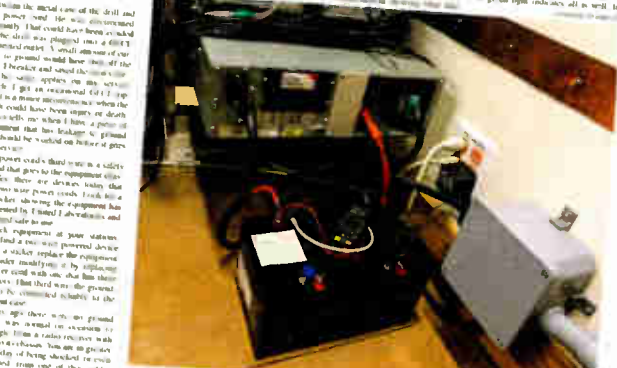
Fig. 2 UPS outlets kept outside the UPS
