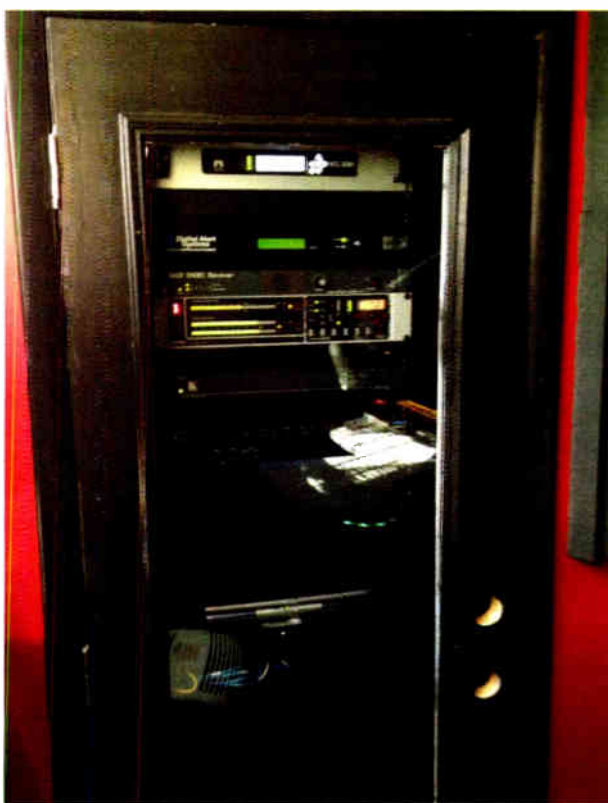
Transmitter rack closet.
