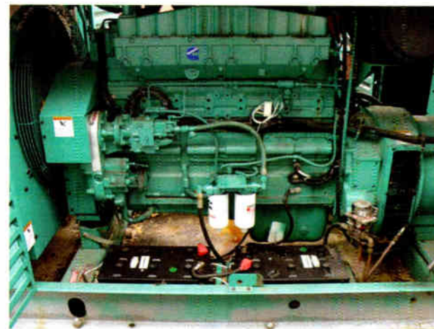
A 100 kW diesel engine at WAWZ(FM).
