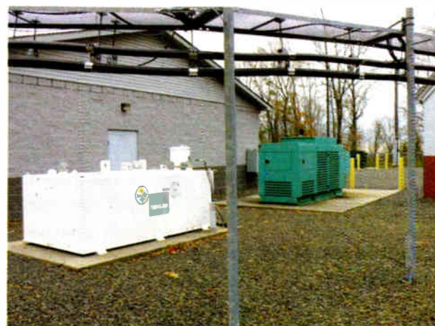
The WAWZ generator, at right, plus tank.
