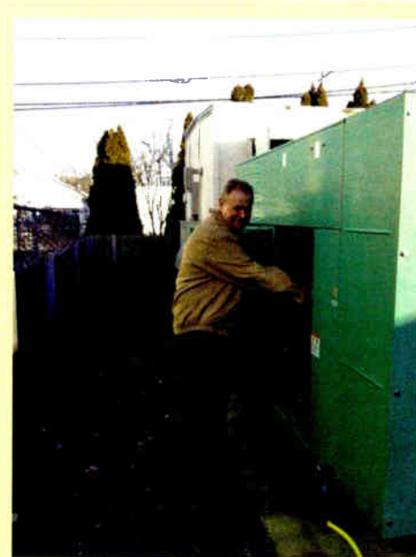
Bill Clanton, station engineer at WRAT(FM), checks up on the genset.
