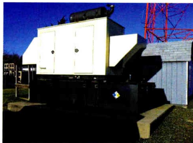
A full 200 kW generator at WCTC(AM)/WMGQ(FM).
