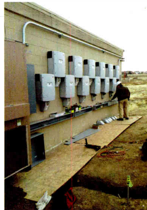
An unidentified technician from REC Solar installs inverters on the wall of the transmitter building.
