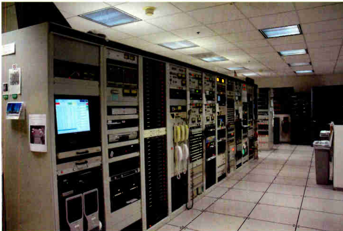
Before: The old rack room.
