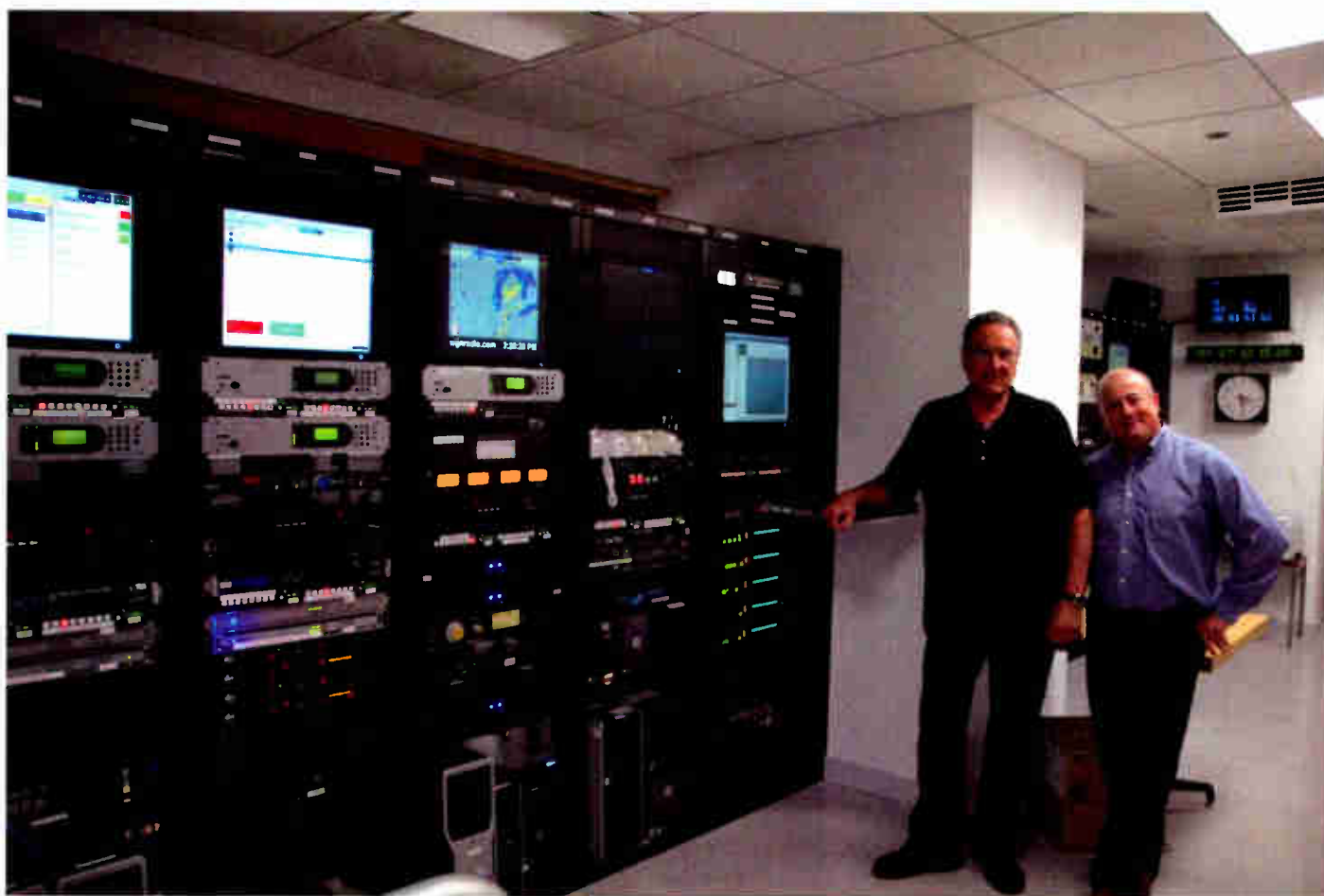
Jim Carollo and former GM Tom Langmyer in the newly completed rack room.
