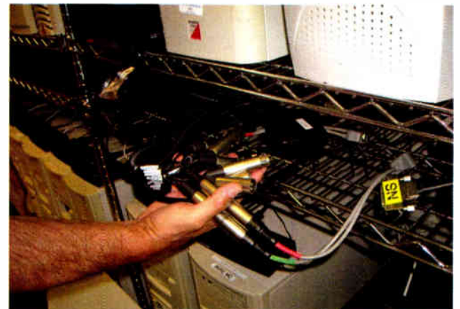
Fig. 4: Smaller shelves under the computers hold wiring.
