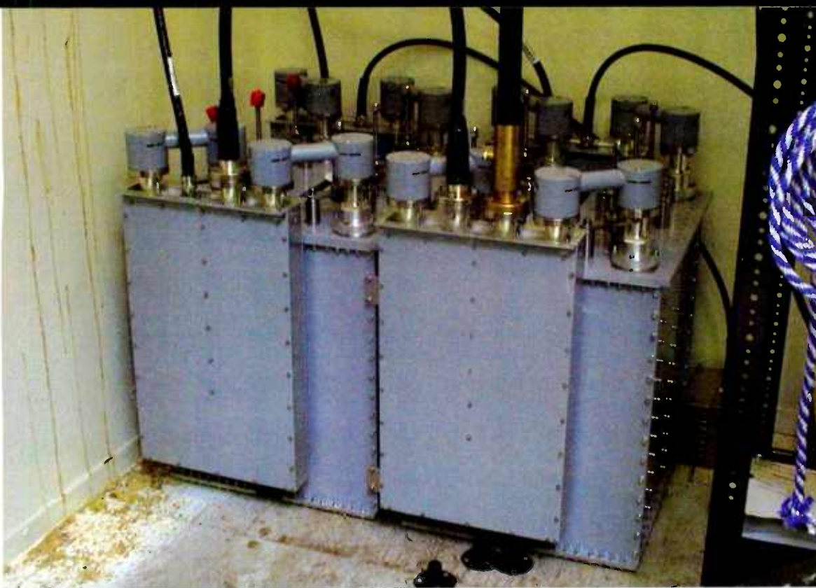
A Bext filter/combiner serves the three translators. Field adjustment was required to get proper performance due to minor adjustment changes that occurred during shipping.
