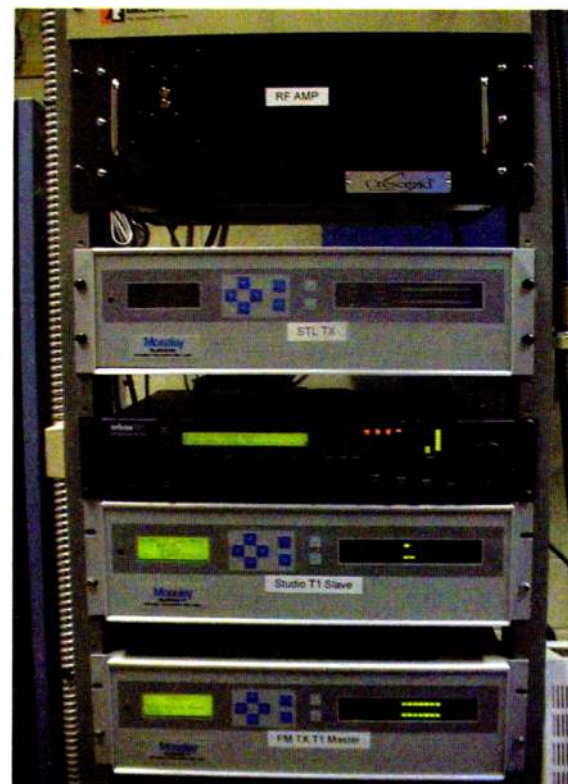
An STL rack at AM transmitter site shows existing Moseley T1 equipment and newly installed second hop for the main FM signal. The new Moseley also transports the Ethernet connection between the studio-mounted HD Importer and Exporter to the HD exciter at the FM transmitter.
