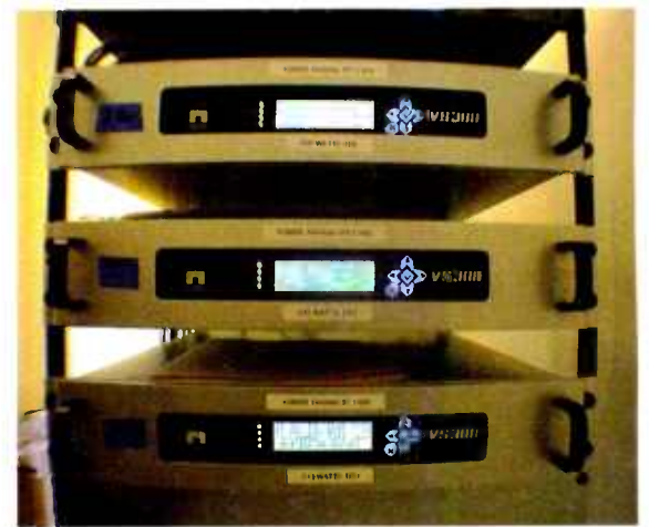
Nautel VS300 transmitters are used for the translators.
