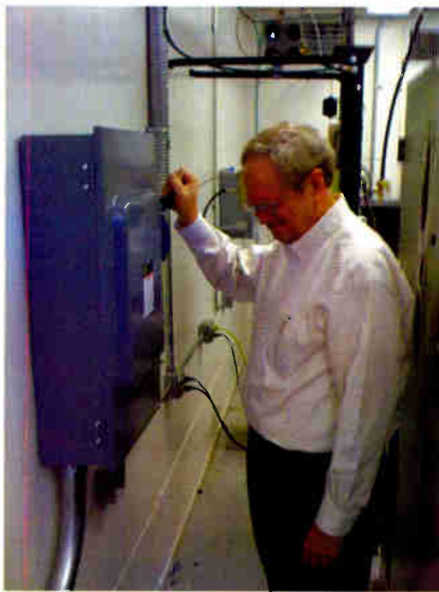
Downs turns on the 200 amp breaker to a new Harris HPX 30 kW transmitter for analog FM and HD Radio for KNDE(FM).
