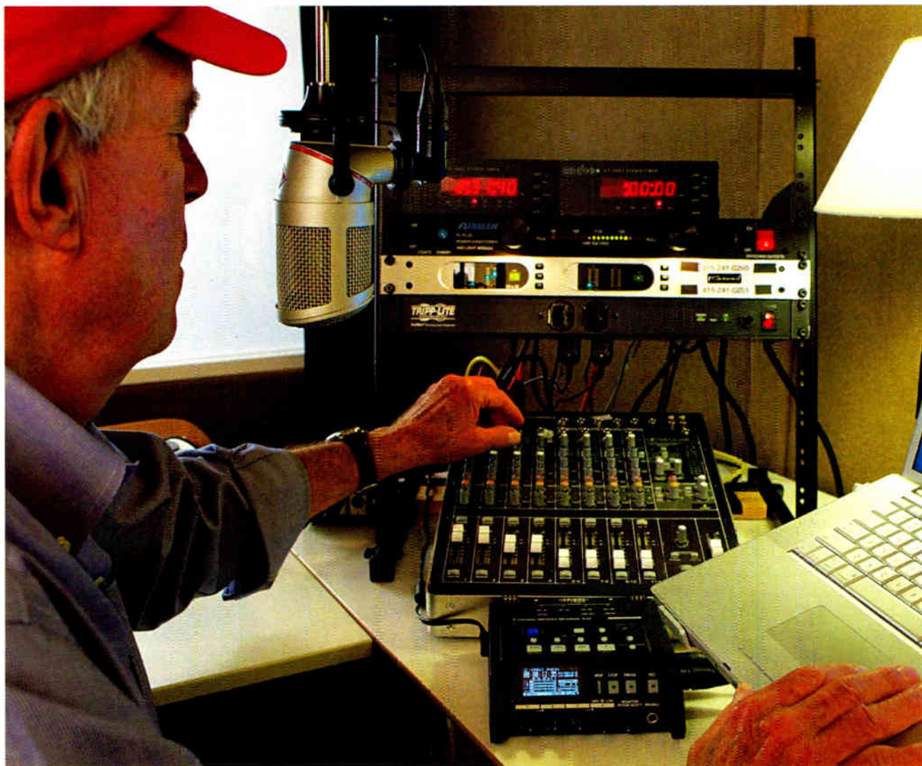
Christopher Springmann drives his rig. The Telos Hx2 is in the rack above the mixer.
