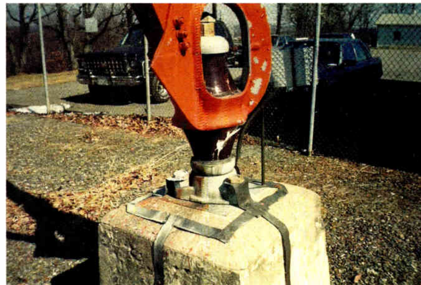
Fig. 4: The damage to the southeast insulator was almost as bad as that suffered by the northeast leg.
