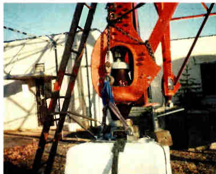
Fig. 2: Here we see Sky Tower Service's temporary repair to support and restrain the northeast leg.
