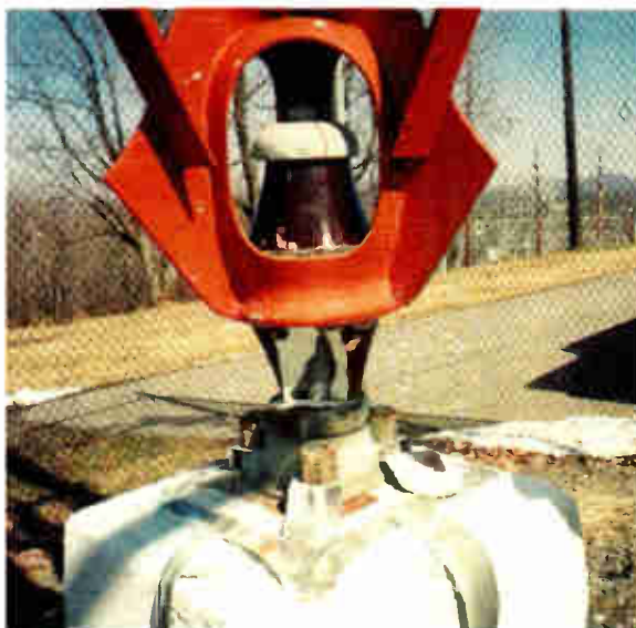
Fig. 1: The insulator on the northeast leg sustained the most serious damage.
