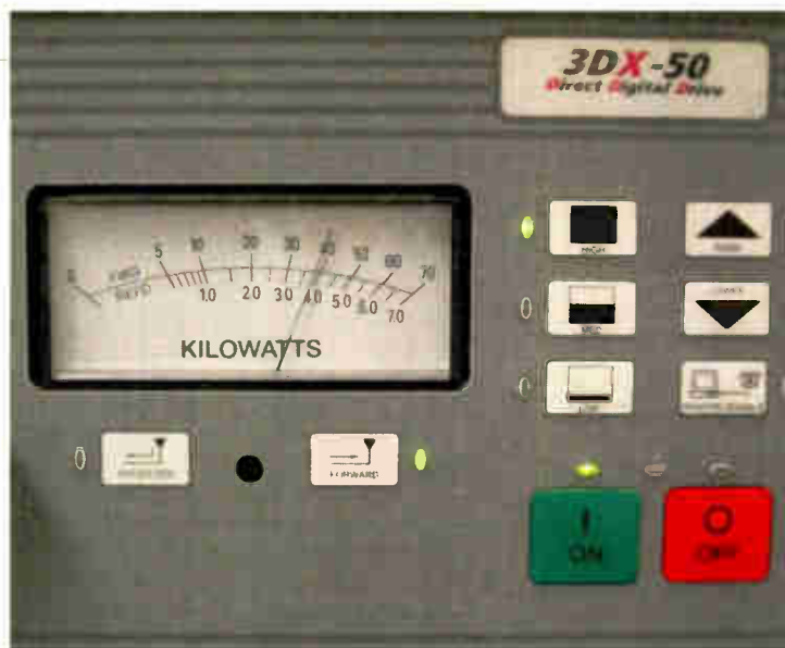
The meter reading of about 38 kW is the approximate average power level reading of a 50 kW transmitter after the AMC (-3 dB) MDCL algorithm was turned on. Normally the meter would read 50 kW.
