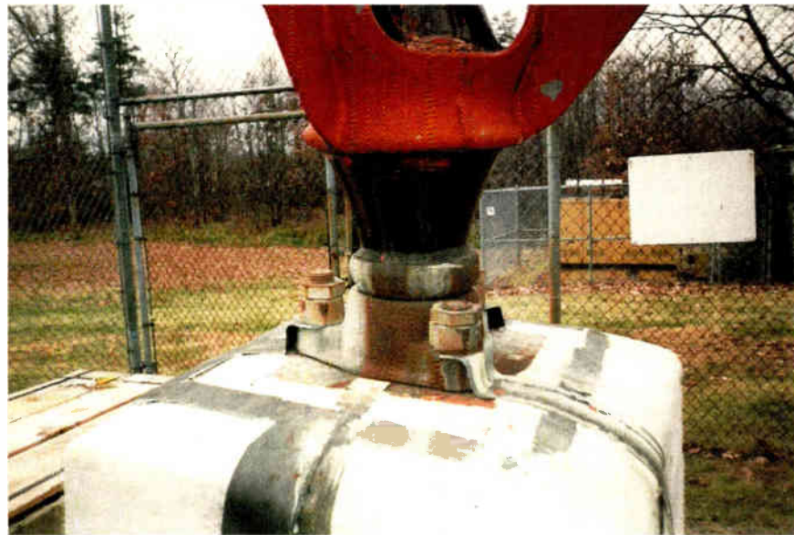
Fig. 3: Porcelain insulators can also crack, as seen in the northwest leg.
