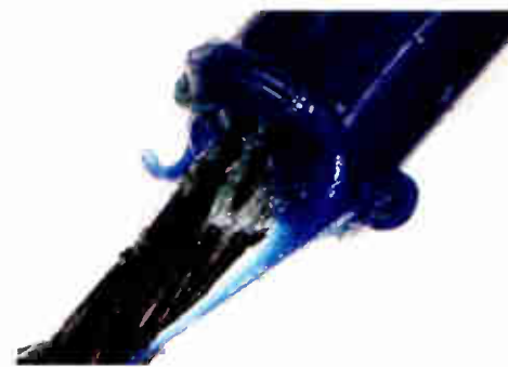
Fig. 3: Remove the wire insulation to see the damage caused by the corrosion.
