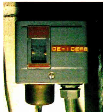
Fig. 2: Check proper operation of deicer controls. It's effort well spent this time of year.
