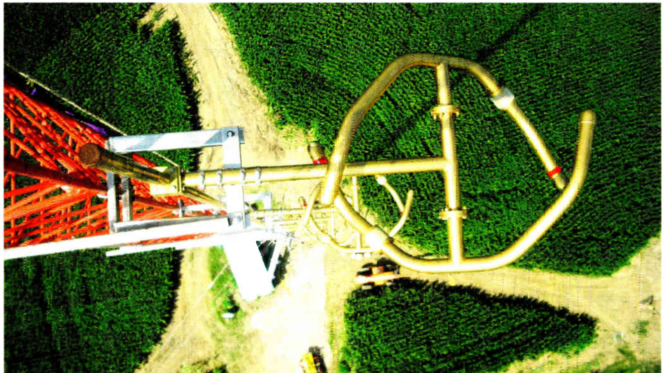
View from the top of WIBN's new 295-foot tower showing the new ERI LPX-6C RotoTiller FM antenna.
