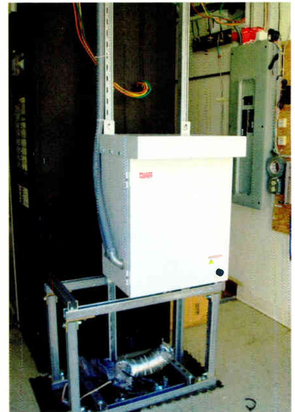
Fig. 2: The Phase Perfect converter, mounted and ready for service.
