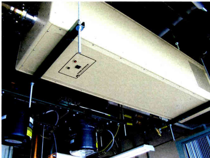
This photo isn't sideways! Working with tight spaces is among the challenges of many transmitter installations these days. WFMT(FM) in Chicago has mounted its dummy load by suspending it from a ceiling. Another trend is greater redundancy built into transmitters. WFMT, using a new Nautel NV40, operates without an aux for that reason.
