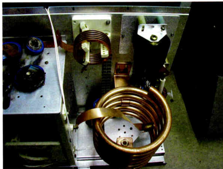
Fig. 1: Destroyed blue capacitors required a novel solution.
